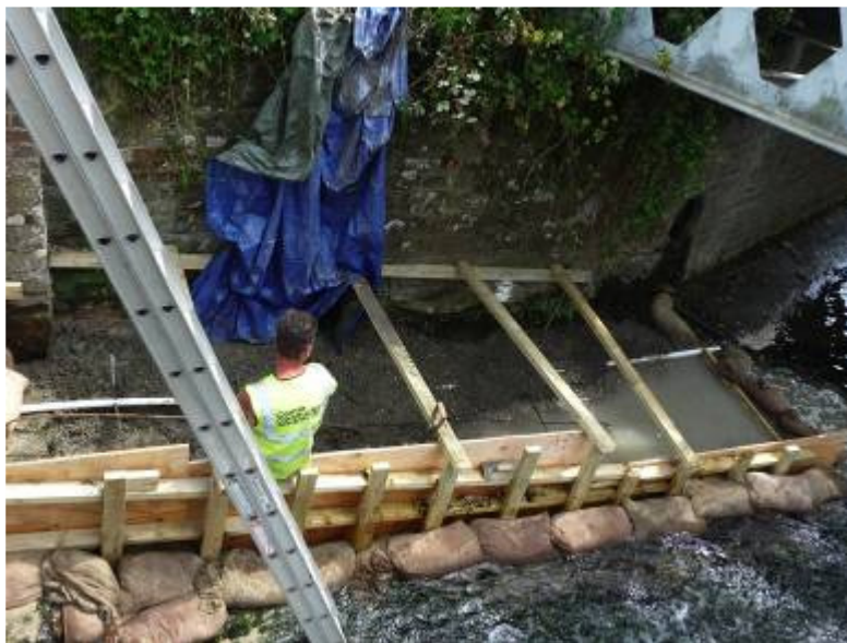
Figure 5: Creating the concrete ramp alongside the bridge wall up to the first hatch
