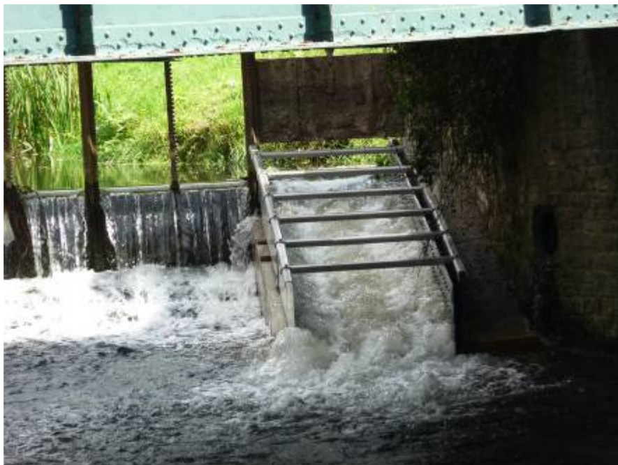
Figure 6: Within an hour the water level had risen sufficiently to come down the fish pass. At first a small trickle then the flow increased
