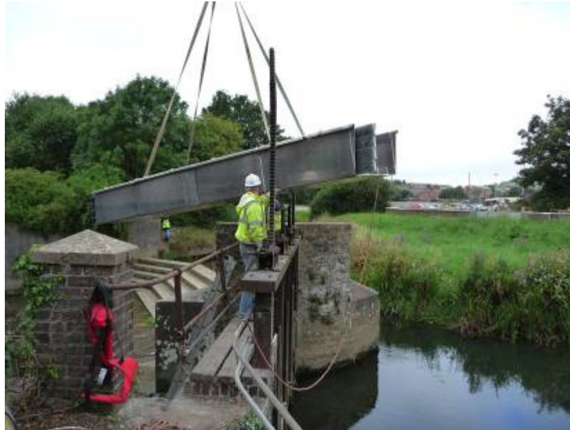
Figure 6: Very tight fit. Using a crane to lower very slowly between the hatch support frame and the power supply pipe.
